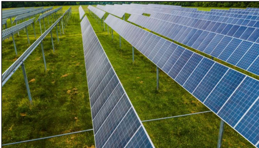
Figure 17: A Typical Operational Solar Farm (Credit: Energy Guide UK 42 )
